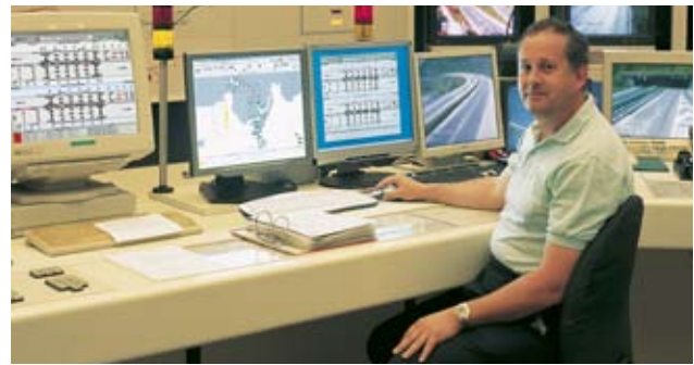
Fig. 1: Jean-Michel Niklaus in the Camorino traffic control center; no alarm goes unnoticed thanks to indicator lamps
